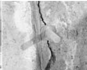
Center port over crack
