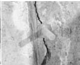
Center port over crack
